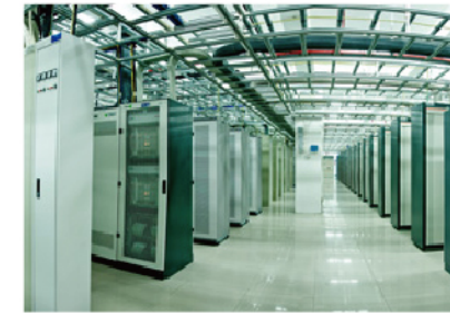
Jilin Mobile Data Center Place: Jilin Area: 10400m 2 Panel Type: Calcium sulphate panel
